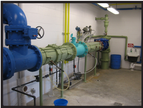
Interior pump house piping for well #11
