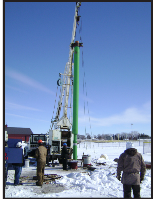
LAKOS PPS Pump Protection Separator during installation in Rochelle, IL
