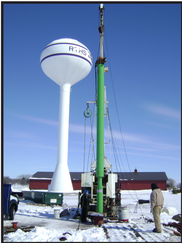
PPS during installation. The separator saved the City of Rochelle hundreds of thousands of dollars in well rehabilitation costs.
