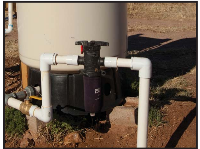
LAKOS TwistIIClean installed downstream of the pressure tank
