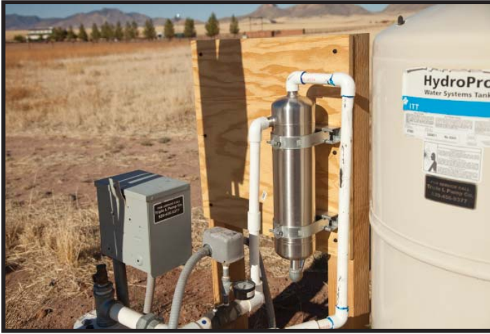
LAKOS SandMaster Plus (stainless steel) installed between the submersible pump and the pressure tank
