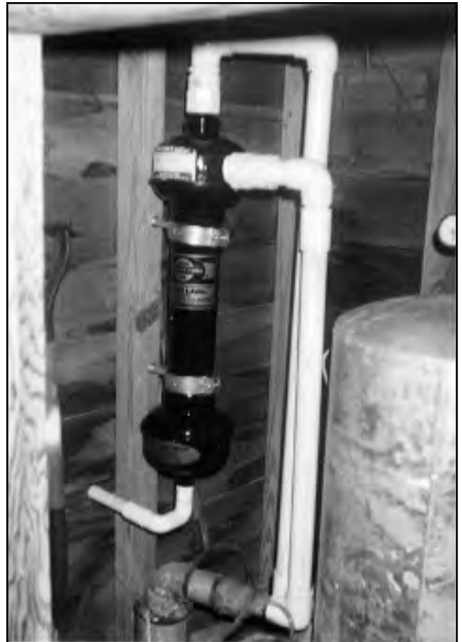
(Above) The LAKOS Separator, installed between the well-head and pressure tank, is totally hidden from view in a picturesque wooden shed that complements Roberts’ Florida lawns and gardens.
